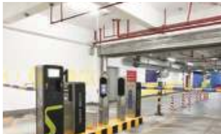
Smart parking system
